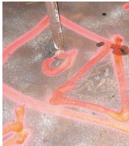
Corroded Tank Floor
